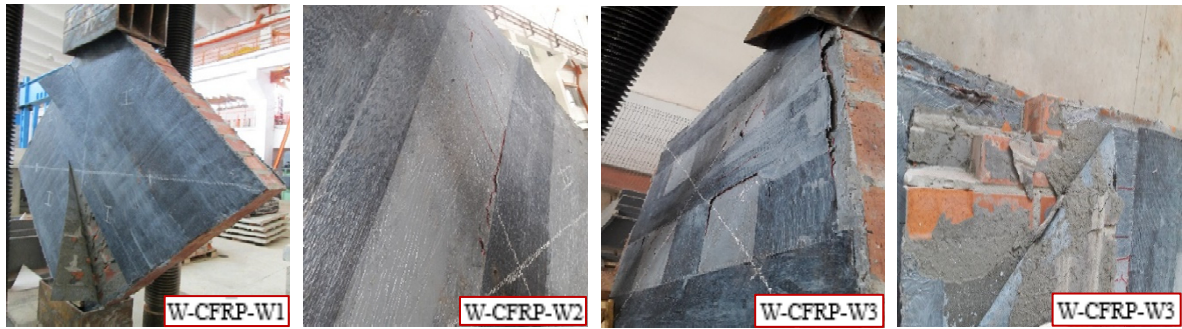
Shear crack formation along the diagonal and the delamination of CFRP (Group N°1)
