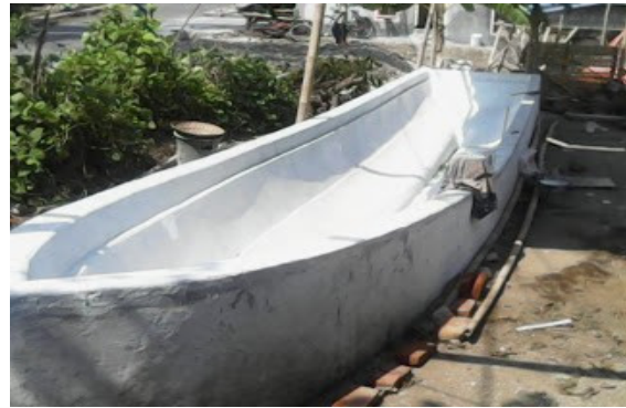
Figure 2: The processing of fiberglass fishing vessel with FRP technology using permanent mold making model role.
