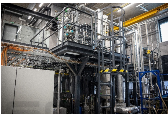
Figure 10: Thermochemical Conversion Laboratory.
