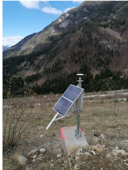
Figure 9: LGMS installed in Gummern.
