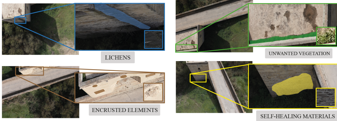
Figure 3: UAV images highlighting the anomalies taken into account in this investigation.
