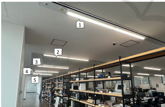
Figure 5: Lighting devices to be verified.
