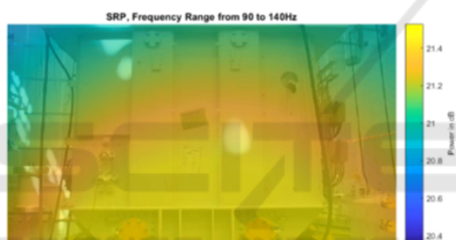
Figure 5: Sound radiation pattern for frequency band 90-140Hz of a transformer.
