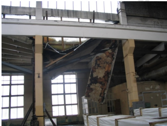
Figure 3: Collapse of industrial building due to incorrect prediction of column foundations settlements.
