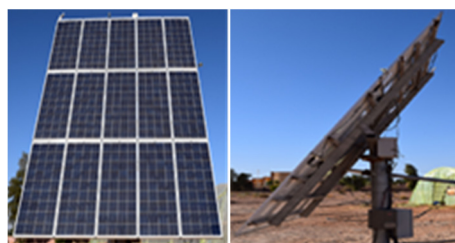
Figure: 1. Photovoltaic system mounted on the sun tracker
