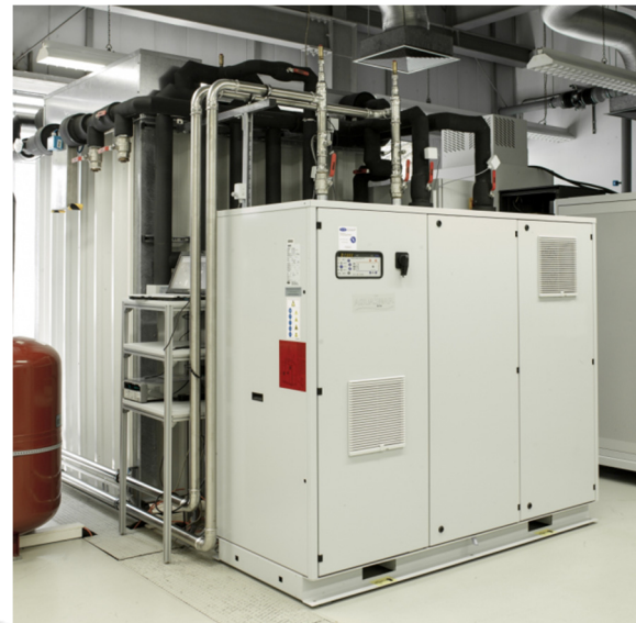
Figure 2: Compression chiller and ice storage system under test.
