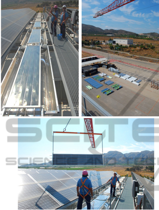
Figure 3: Solar thermal cooling-heating system: Installation process and collecting surfaces.
