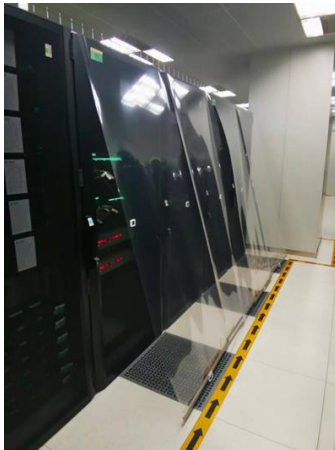
Figure 15: Continuous air curtain in front of the F02-F05 cabinets.
