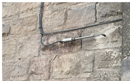
Figure 4: Instrumental crack monitoring system on a listed building.
