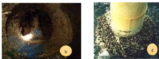
Figure 1. Marine growth and its effects, (a) intake hole, (b) pipe interior, (c) filter, (d) pole base plate
