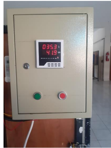
Figure 2: Thermostat and humiditystat installed on the Smart control panel.
