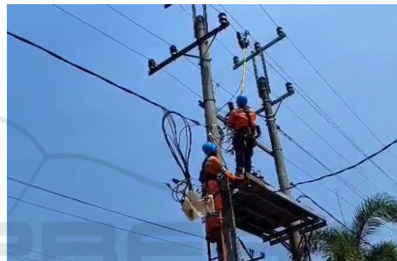
Figure 8: Barong install the Insulator Cover on Live Line in Udiklat PLN Semarang Center Java.
