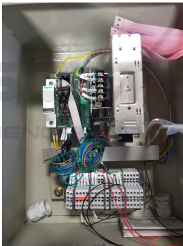
Figure 2: Control panel wiring.
