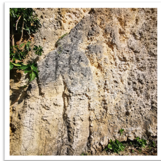
Figure 5: Crack or discontinuities condition on the rock mass in Melasti Beach area.
