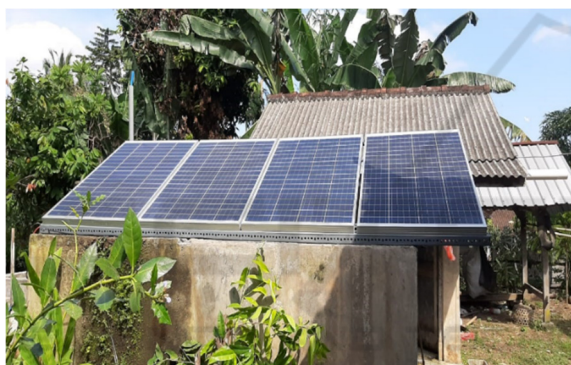
Figure 4: Solar panel used to energy source.
