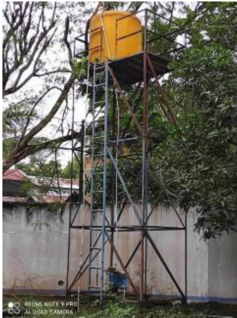
Figure 2: The Pico-Hydropower System.
