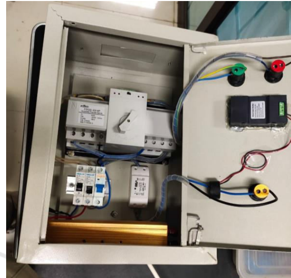
Figure 6: Auto Transfer Switch Panel.
