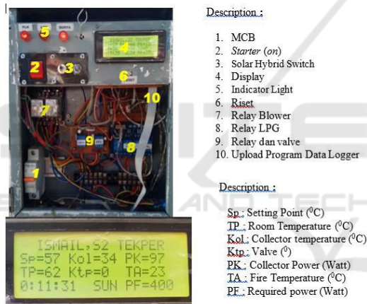
Figure 9: Dryer Control Point.
