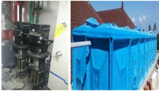
Figure 8: Installation of a clean water supply system and tower tank at Luna 2 Hotel Seminyak.
