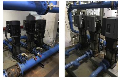
Figure 5: The installation of a clean supply system at Double-Six.Luxury Hotel Seminyak uses 3 pumps.
