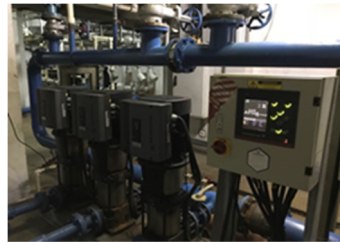
Figure 6: Control Panel of the clean water supply system at Double-Six Luxury Hotel Seminyak.
