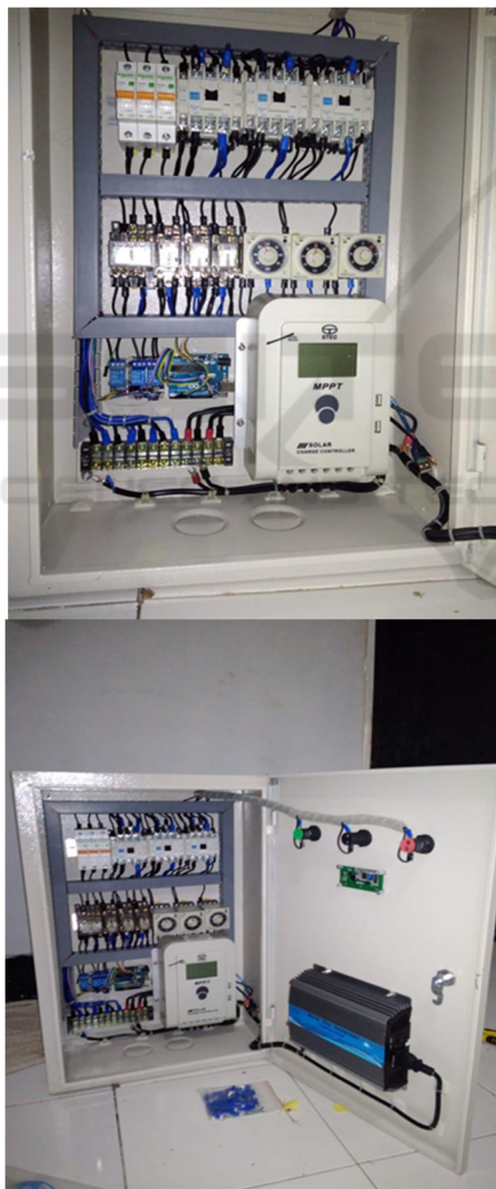
Figure 8: System Electricity Smart Controller SHS for Load Management.
