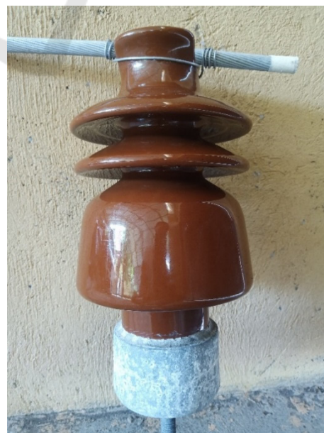
Figure 8: Pedestal insulator on clean and dry.
