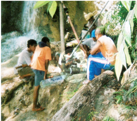
Figure 3: Operating 3-inch Hydraulic Ram pump.
