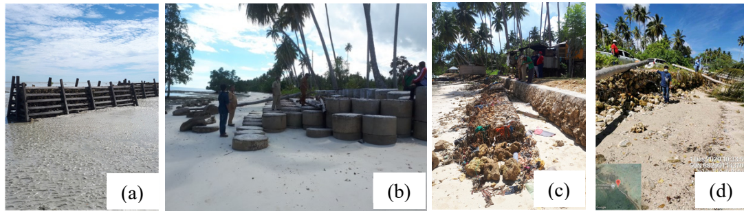
Figure 3: Simple coastal protection structures on the shoreline of Biduk-Biduk: (a) breakwater, b) concrete-ring revetment, c) rock revetment, d) gabion.
