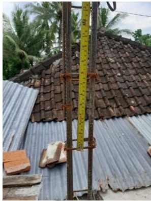
Figure 3: The details of the distribution reinforcement do not meet the requirements.
