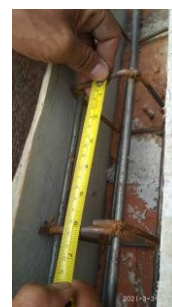
Figure 2: Plain reinforcement and wide stirrups.
