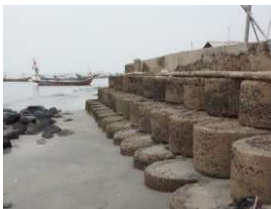
Figure 2: Sedimentation and coastal structure damages.
